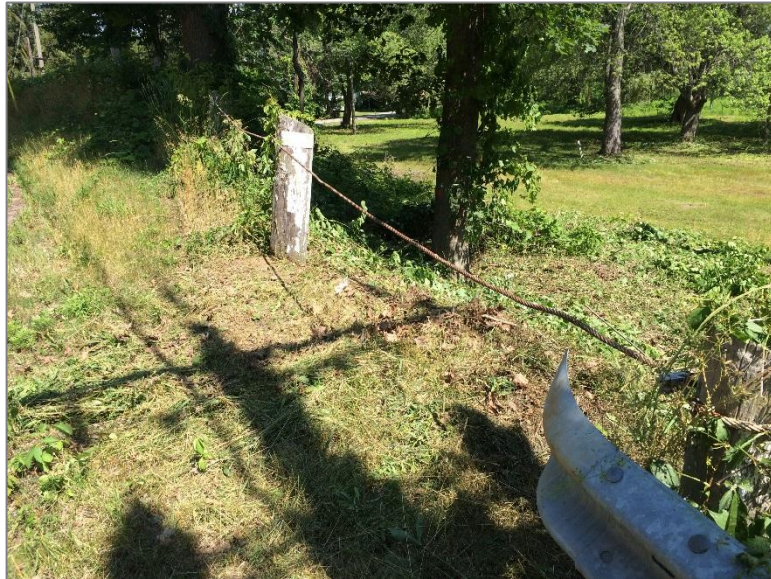
Figure 3-4 Design Conformance Issues (Lakeshore Road)
