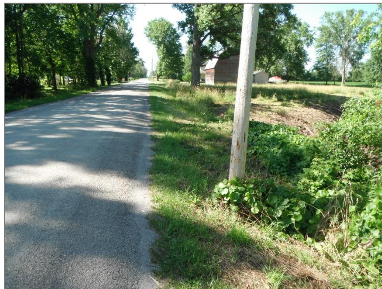
Figure 3-2 Fully-Unprotected Hazard (Prestman Road)
