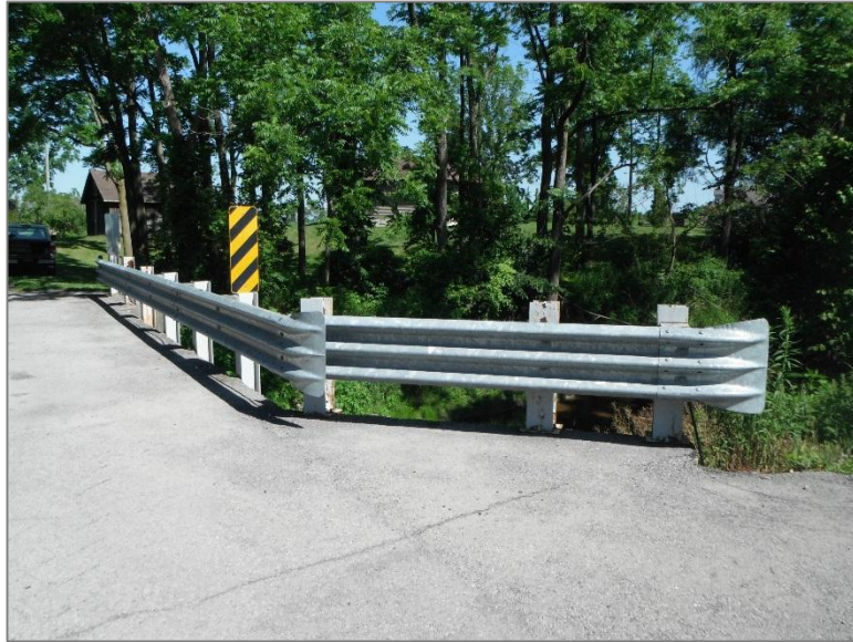
Figure 3-5 Design Conformance Issues (Mill Race Road)
