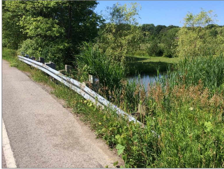
Figure 3-3 Partially Protected Hazard (Cement Road)
